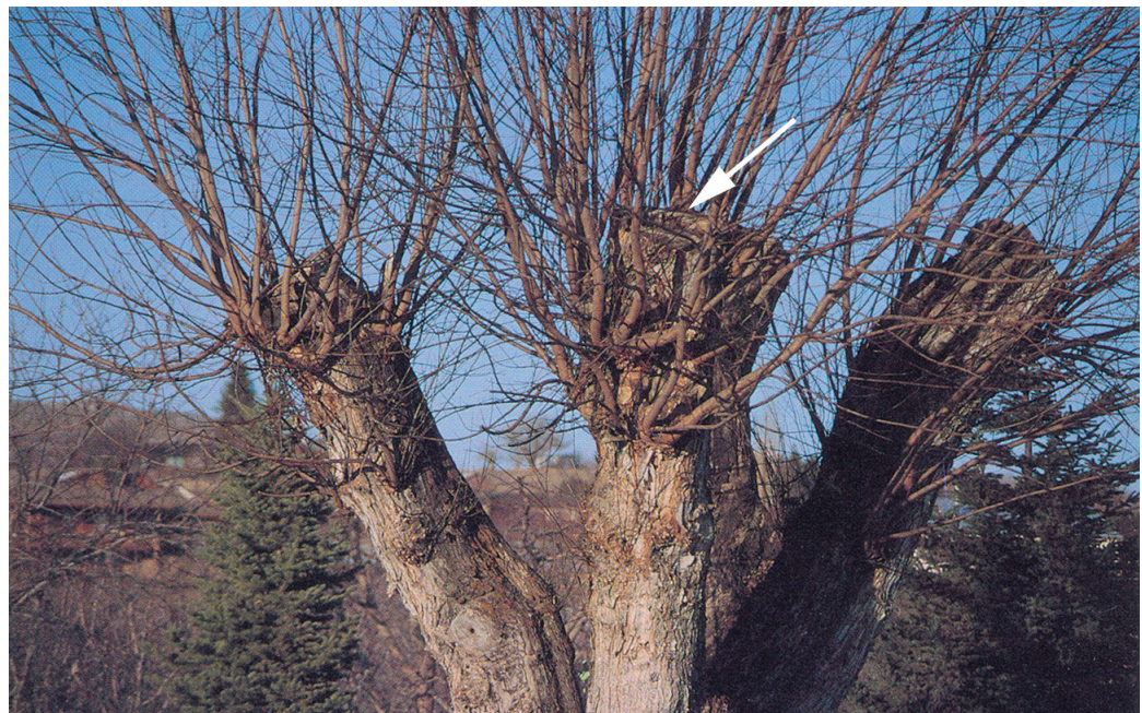
Figure 5. The heading or stub cuts of these large limbs have led to vigorous new growth. The tree also has been severely disfigured by this type of pruning. (Heart rot evident at arrow).
