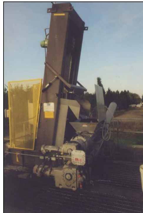
Mechanically raked bar screen and washer/compactor.
