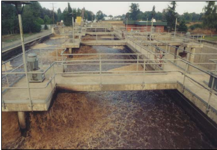
Aeration basin and surface aerators.
