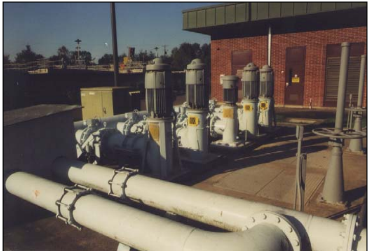
Vertical turbine effluent pumps.
