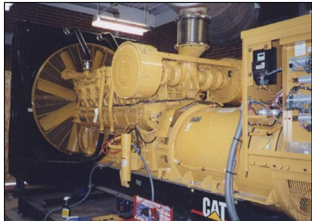
Standby generator system.
