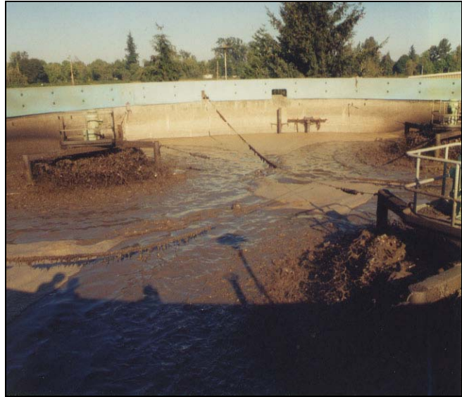
Large aerobic digester with surface aerators.
