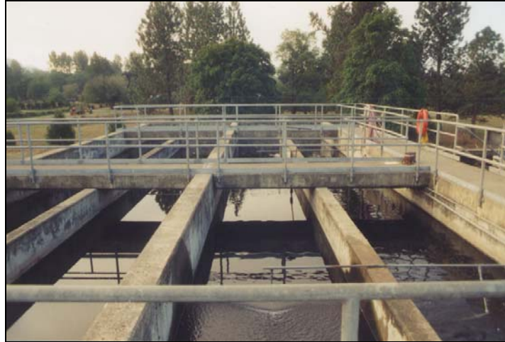
Chlorine contact tanks.
