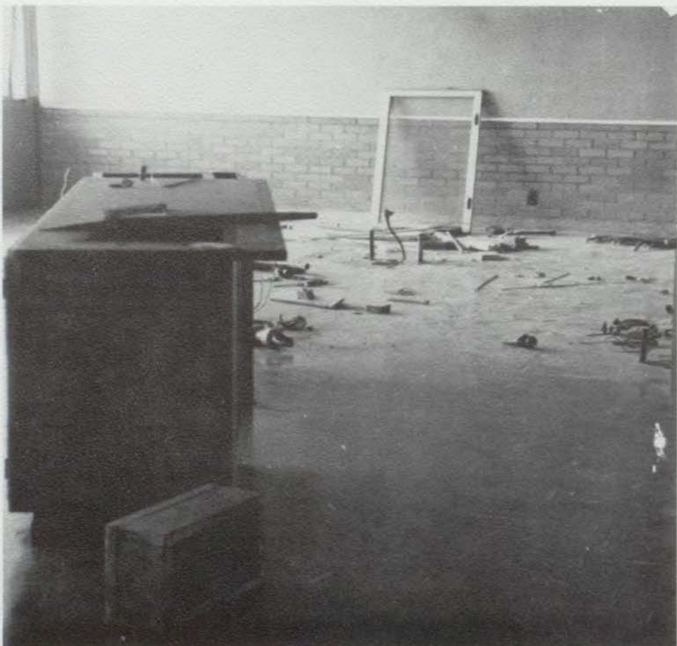
Maintenance men worked on the chemistry room looking for a gas leak.
