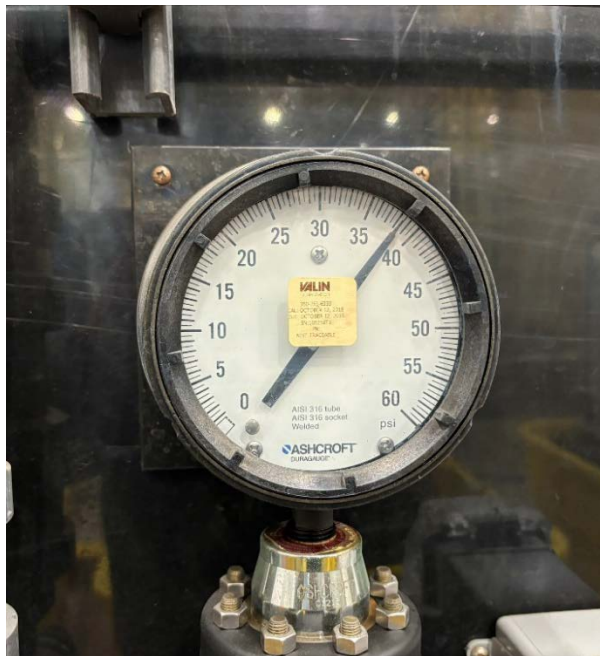
Pressure Gauge – Inside Water Treatment Plant
