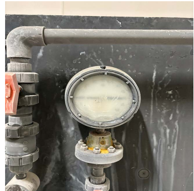
Pressure Gauge – Inside Fluoride Containment Room
