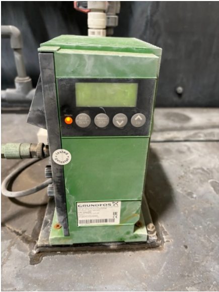
Inside Fluoride Containment Room
