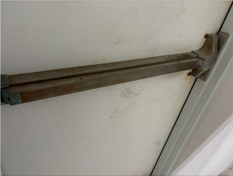
Standard Door Handle – Inside Fluoride Containment Room
