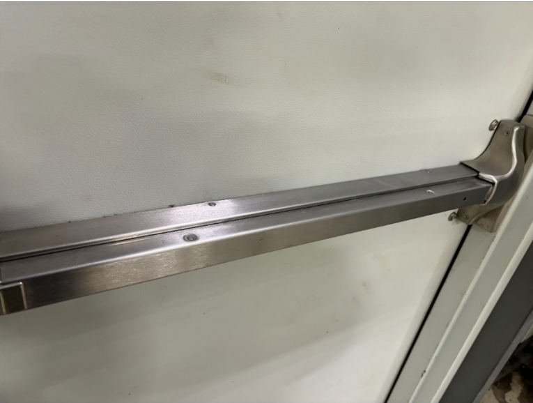
Standard Door Handle – Inside Water Treatment Plant
