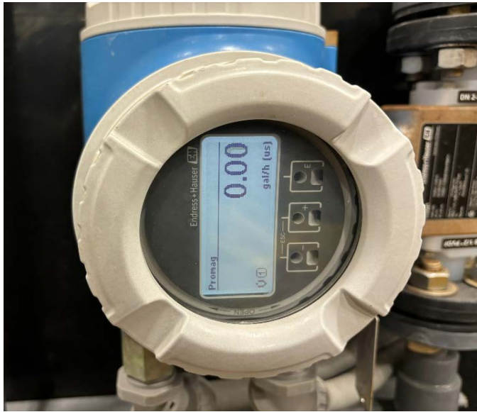
Flow Meter – Inside Water Treatment Plant
