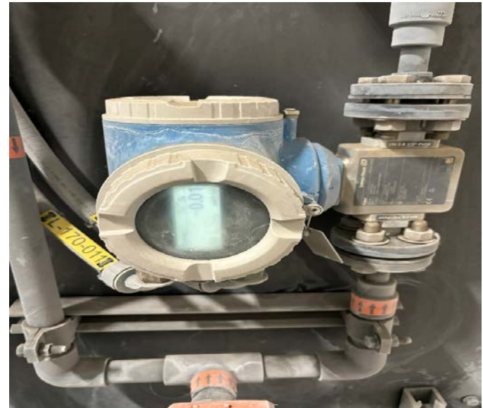
Flow Meter – Inside Fluoride Containment Room
